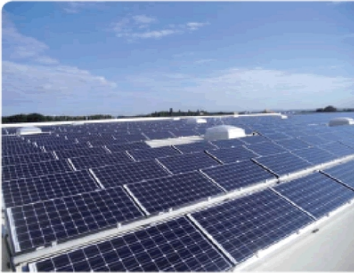
Self consumption of green solar generated energy
